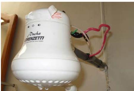
Figure 20.41 On-demand electric hot water heater. Heat is supplied to water only when needed. (credit: avidavid, Flickr)
