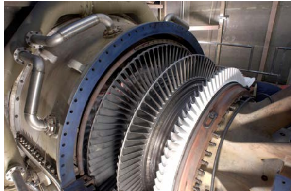
Figure 23.24 Steam turbine/generator. The steam produced by burning coal impacts the turbine blades, turning the shaft which is connected to the generator. (credit: Nabonaco, Wikimedia Commons)
