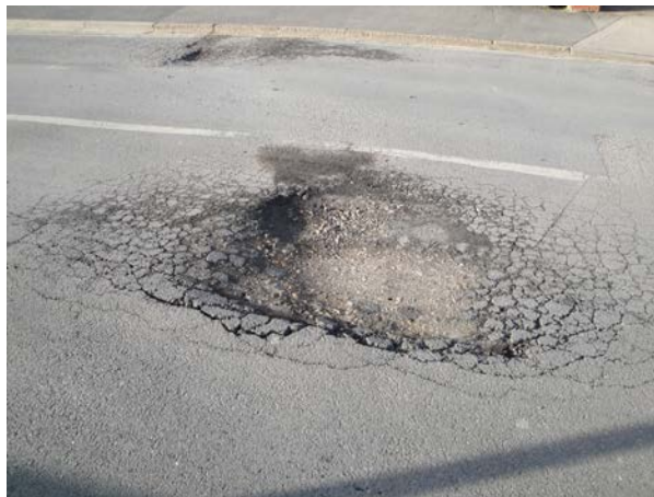
Figure 13.14 Thermal stress contributes to the formation of potholes. (credit: Editor5807, Wikimedia Commons)
